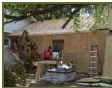
Cornerstone Builders, Inc. connect the buildings at the corner of Moore and Davis Streets
